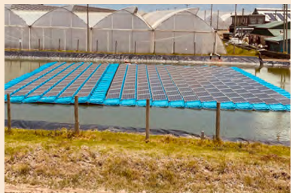
Floating solar plant
